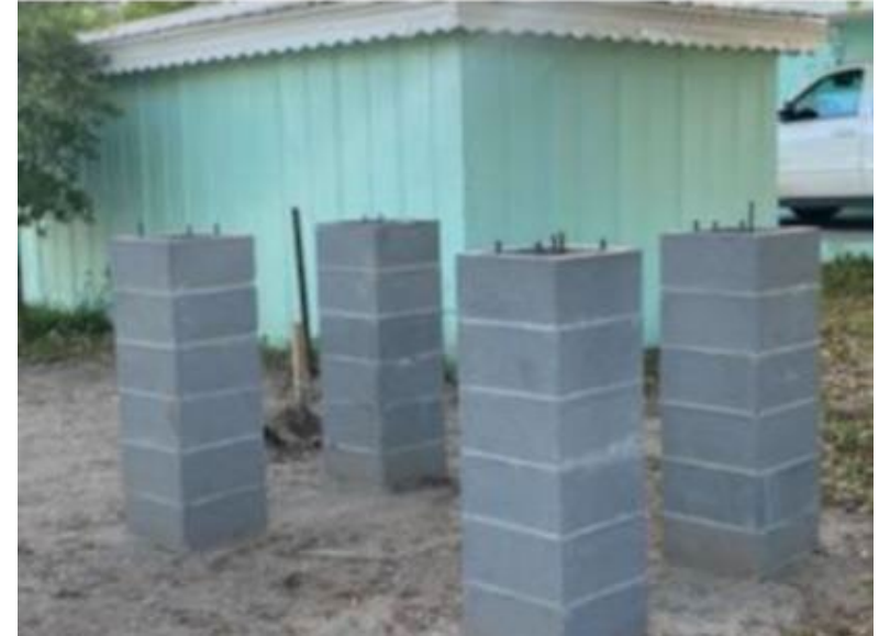
Per FEMA Requirements Generators Must Be Installed Above The Flood Plain.
