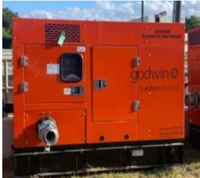
Close-Up Of One Of The Back Up Generators
