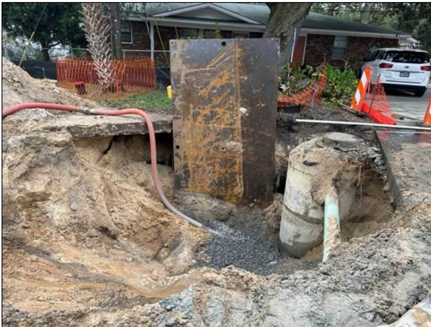
Construction activity at the start of the project at Van Horn and Taylor.
